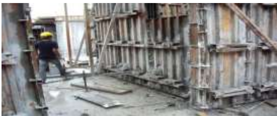
Loss of cement paste through form joints
