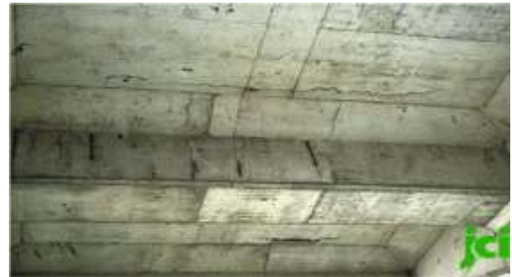
Lack of concrete cover – Cracks occur along the steel bar
