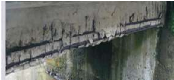
Corrosion of embedded steel due to chloride attack
