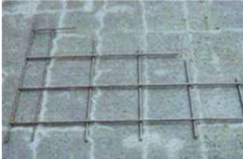
Figure 5. Typical plastic settlement crack
