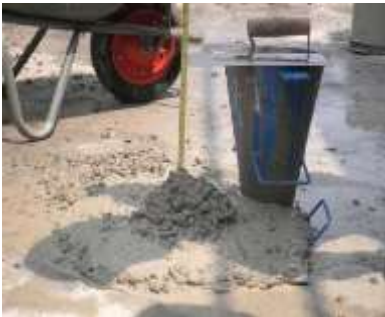
Indication of concrete segregation during slump
