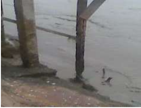
Corrosion of reinforcement
