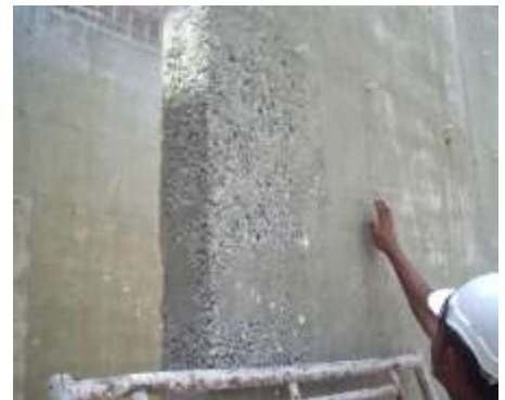
Hardened concrete defect (Honeycomb) due to concrete segregation
