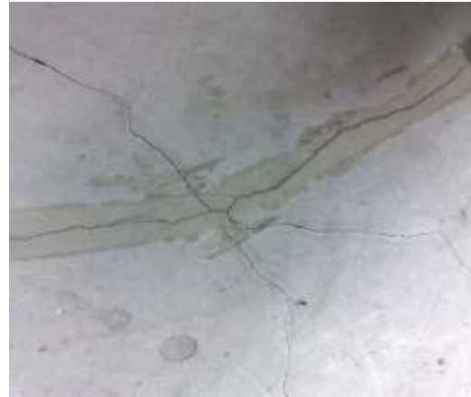
Drying shrinkage crack
