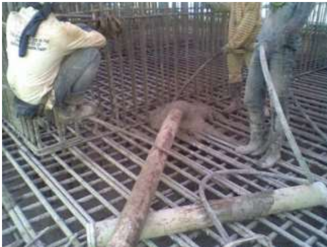
Figure 2. Concrete Pump Blockage at Construction Site
